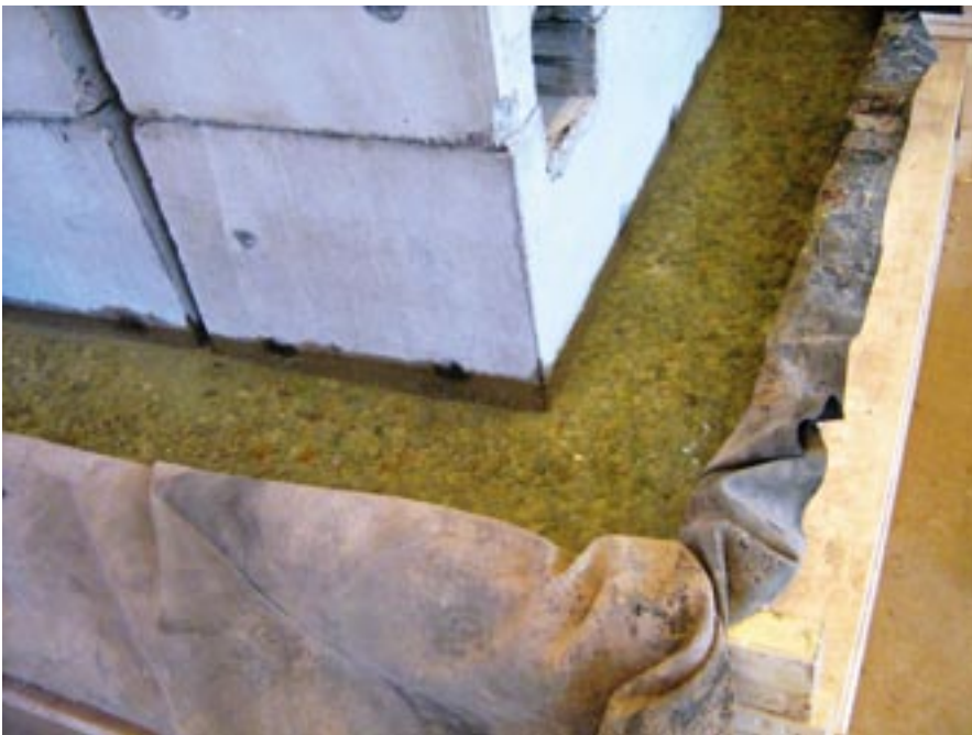
Figure 4-4 Water was standing on the bentonite surface around the piled blocks.
