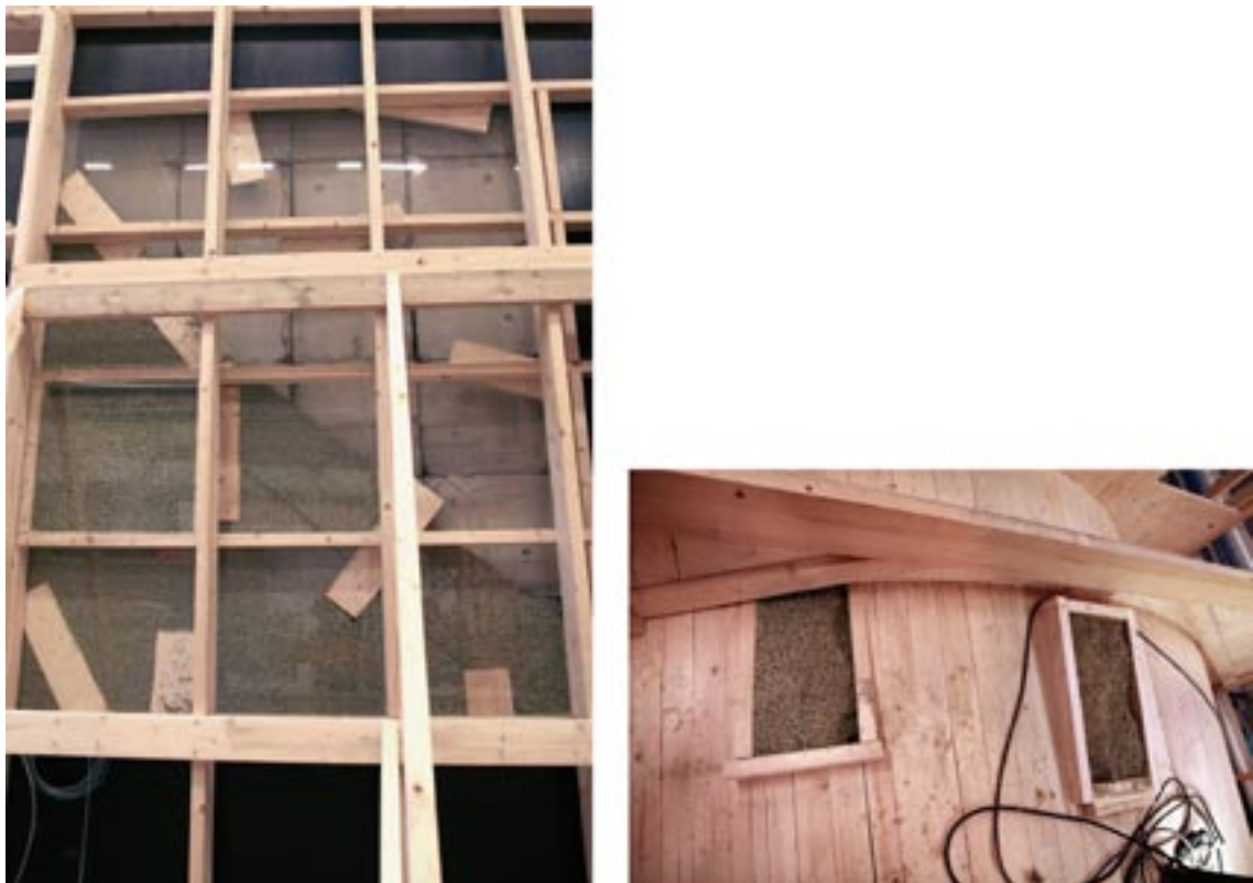
Figure 4-14. Windows for watching motion of pellets and degree of pellet filling.
