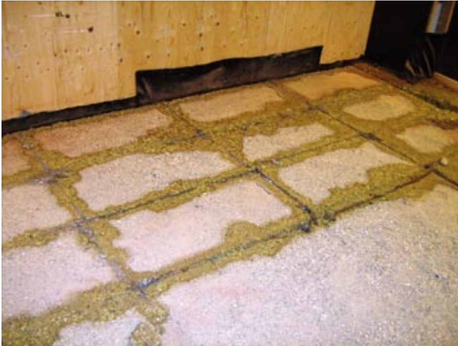
Figure 5-2 After removal of the blocks large dry areas could be seen. Water had flowed between the joints and wet the bentonite.
