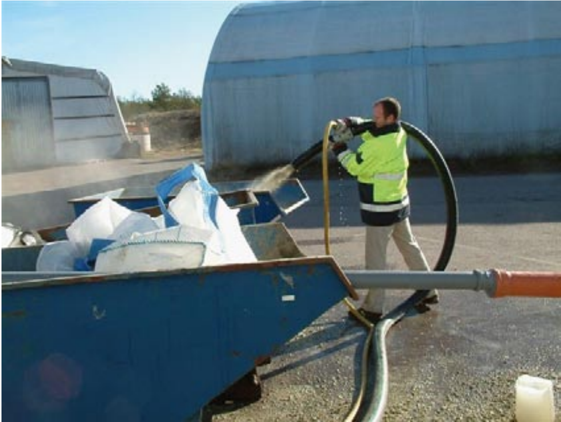
Figure 4-10. Blowing of pellets with a capacity of 1 m 3 /min as part of a study for finding a suitable technique for pellet filling.
