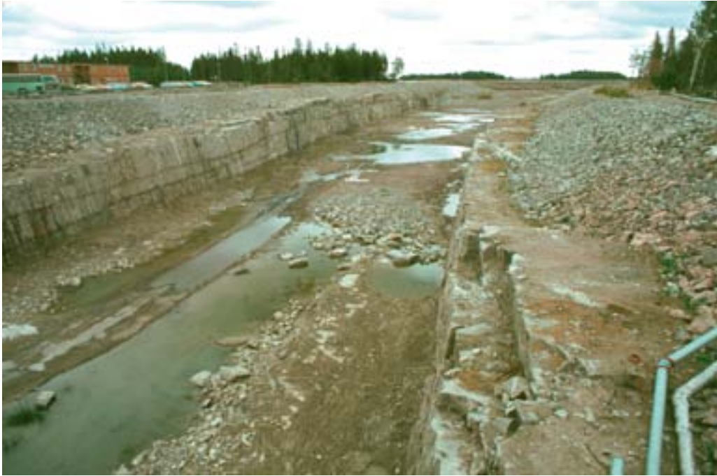
Figure 8-24. Picture from the construction of the 13 m deep and more than one kilometre long canal between the Baltic Sea and the nuclear power reactors in Forsmark. Horizontal fractures/sheet joints are encountered along the entire excavation. The sheet joints follow the undulations of the bedrock surface implying that many of them do not outcrop, but stay below the bedrock surface as this dips under the Baltic Sea. There are several “horizons” of extensive sheet joints on top of each other according to the hydraulic interference tests. The picture is taken from the southern side of the canal where the bridge crosses the canal between drill sites 7 and 8. /Photograph by G Hansson/.
