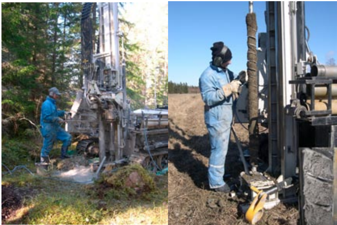
Figure 3-8. Left) A majority of the HFM drillings were performed using percussion drilling. The samples retrieved are often crushed and may include some fragments from the bedrock. Right) At the installation of groundwater monitoring wells (SFM-sites), corings were performed using an auger drill. The coring sites are distributed within the investigation area and resulted in samples of higher quality than from the percussion corer. The picture shows clayey till obtained from 4 m depth at Storskäret. Note the detail in the bottom right hand corner.
