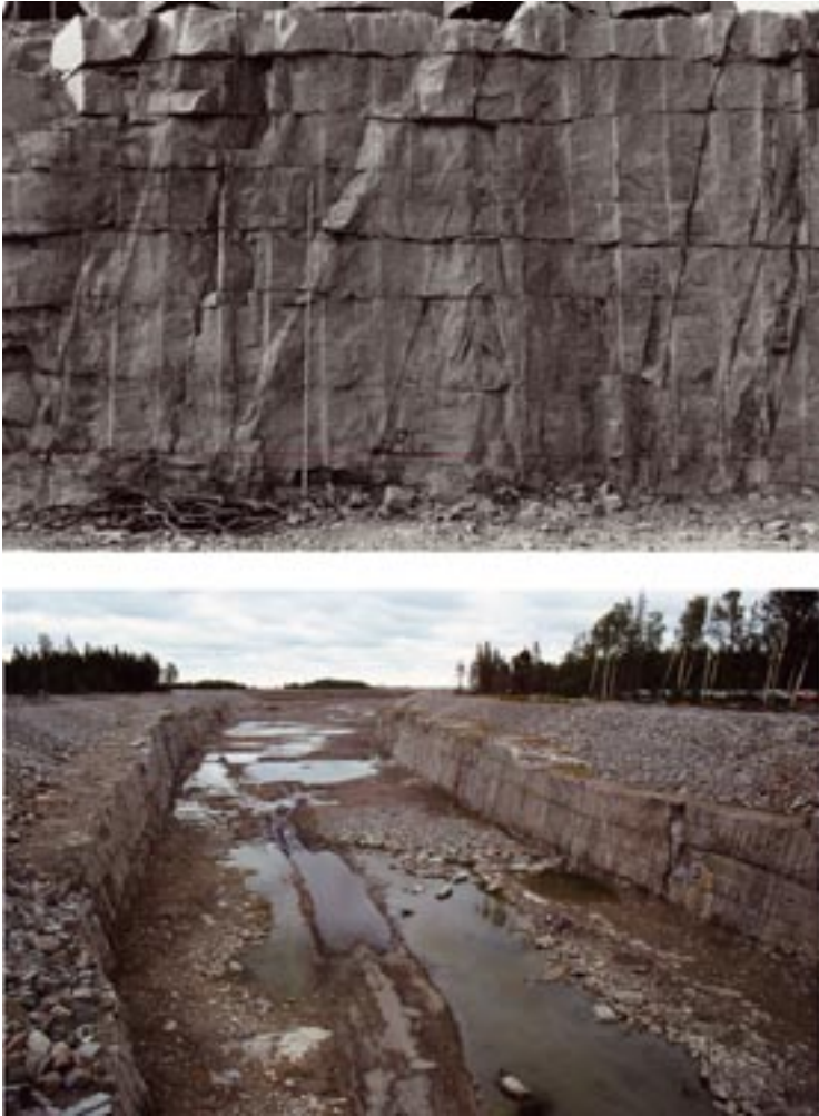
Figure 5-10. Observed near-horizontal and subvertical fracturing in near-surface rock along the Forsmark cooling water inlet canal. Pictures reproduced from /Martin 2007/.
