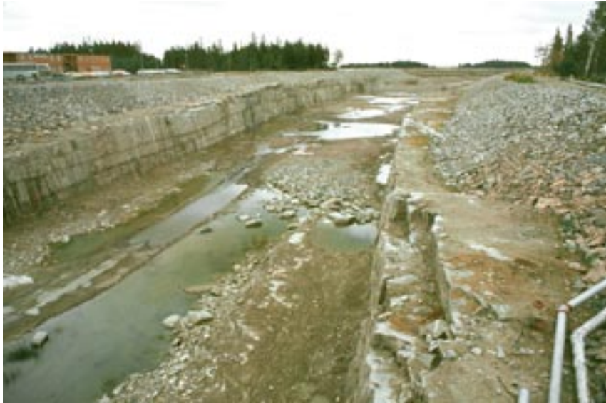
Figure 3-16. Picture from the construction of the 13 m deep and more than one kilometre long canal between the Baltic Sea and the nuclear power reactors in Forsmark. Horizontal fractures/sheet joints are encountered along the entire excavation. The sheet joints follow the undulations of the bedrock surface. There are probably several “horizons” of extensive sheet joints on top of each other according to the hydraulic interference tests. /Photograph by G Hansson/.
