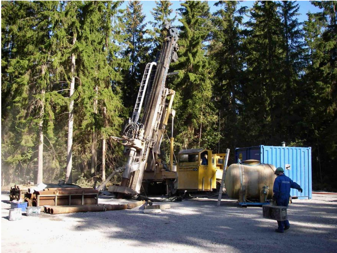
Figure 4-1. The Comacchio MC1500 drill rig performing NO-X 280 drilling through the overburden at KLX21B.
