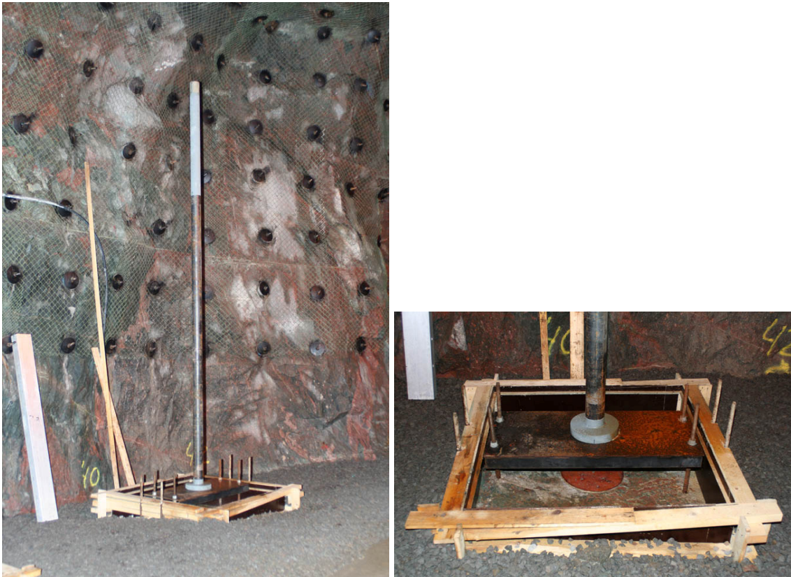
Figure 13. The steel pipe mounted above the deposit hole. The pipe is secured on top of a steel plate. The wooden construction around the deposit hole is the mould for the concrete block that will hold the package in position during the experiment.
