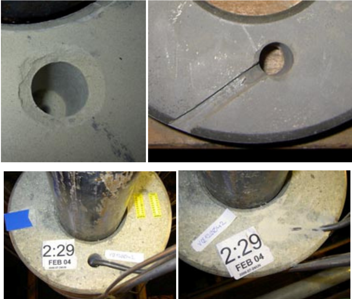
Figure 7. Installation of a RH sensor. Upper left image shows the hole the sensor is installed in. Upper right is the hole and cable notch in the buffer block above the sensor block. Lower left shows a RH sensor installed in the blocks and finally the lower right image shows the completed installation after the hole and notch are filled with bentonite powder.
