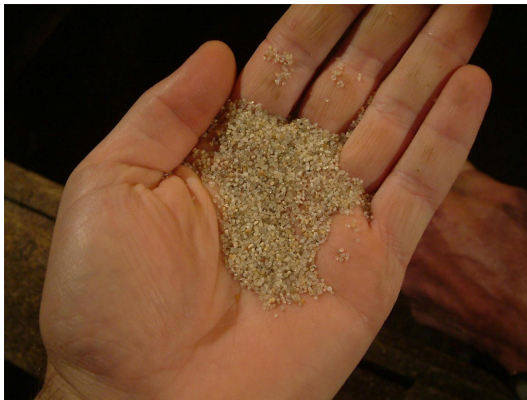
Figure 18. The sand used to fill the slot between the package and rock wall during installation of the second and third package. The sand contains grains of only one size which reduces the risk of lumps forming during the work. The sand will distribute water from both the saturation system and the natural fractures along the packages.
