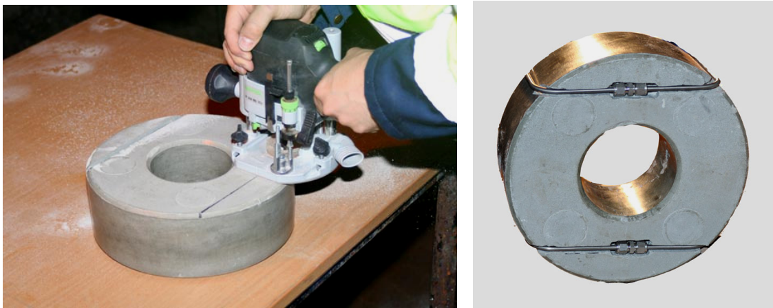
Figure 14. Notches for the saturation system pipes are being prepared in the first block to be mounted in the steel pipe. The notches are cut using a router, left image. The right image shows the completed result with the saturation pipes in position (though without the sand protector around the pipes).
