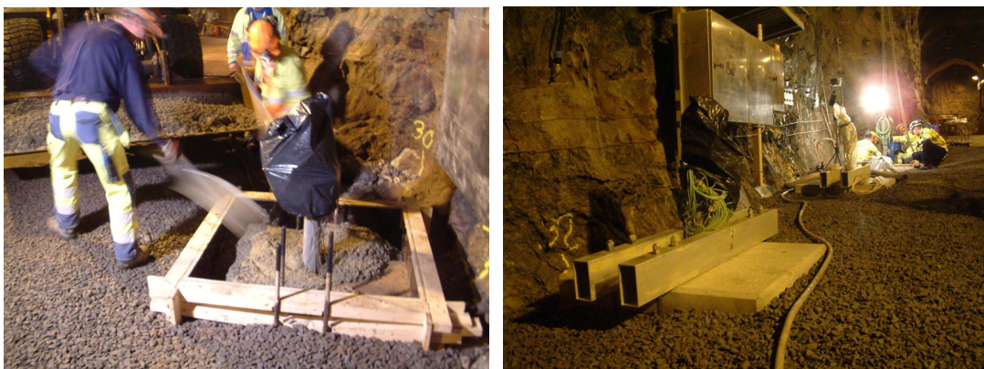
Figure 20. Left: Casting of the concrete block holding the package in place. Right: The concrete block is completed and the two supporting bars are in position. The package installation is completed.
