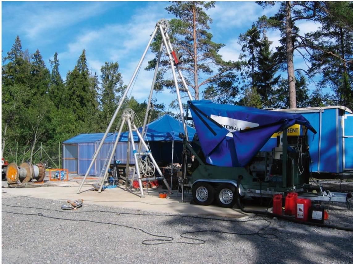
Figure 3-1. Photo of the upgraded MKW wireline unit of Vattenfall Power Consultant AB during operation in borehole KFM08A.
