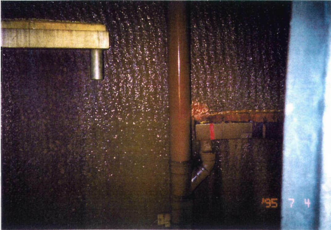
Figure 4-11 Collection of water in the lift shaft.
