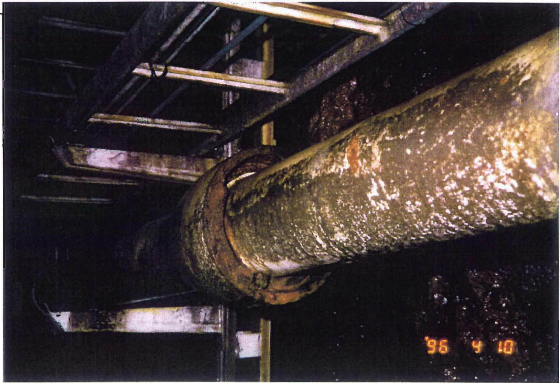
Figure 4-25 Corrosion damaged joint on a VRS-pipe.
