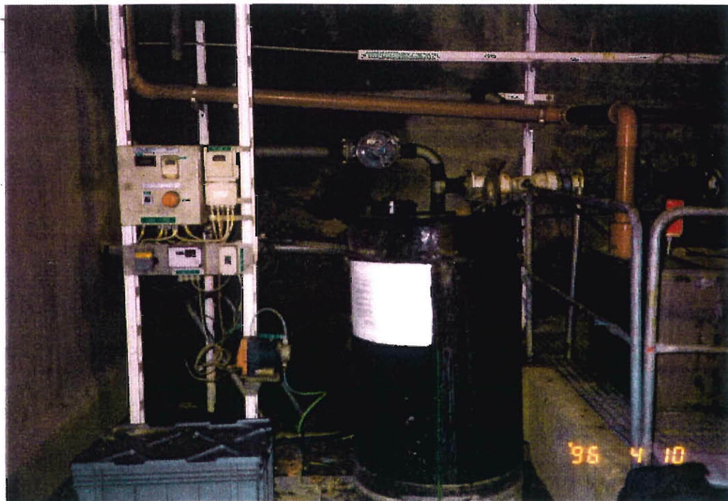
Figure 4-19 Uranine dosage equipment.
