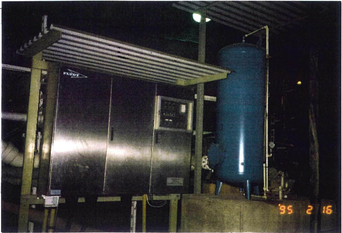
Figure 4-14 Pent-roofs and pressure tank at PG3.
