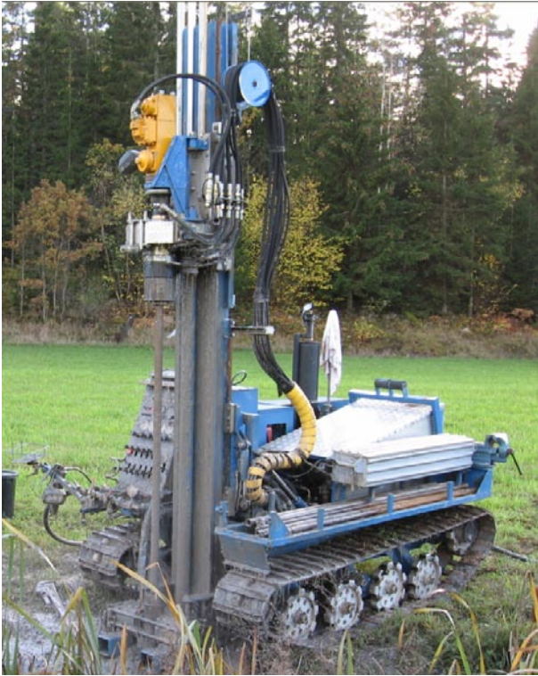
Figure 3-2. Drilling rig HAFO 1500 was mainly used for soil-rock probing, soil sampling and installation of groundwater wells.
