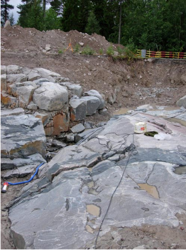
Figure B-1. View of the excavated area from the east. Note the difference in the fracture pattern N and S of the trench, respectively.
