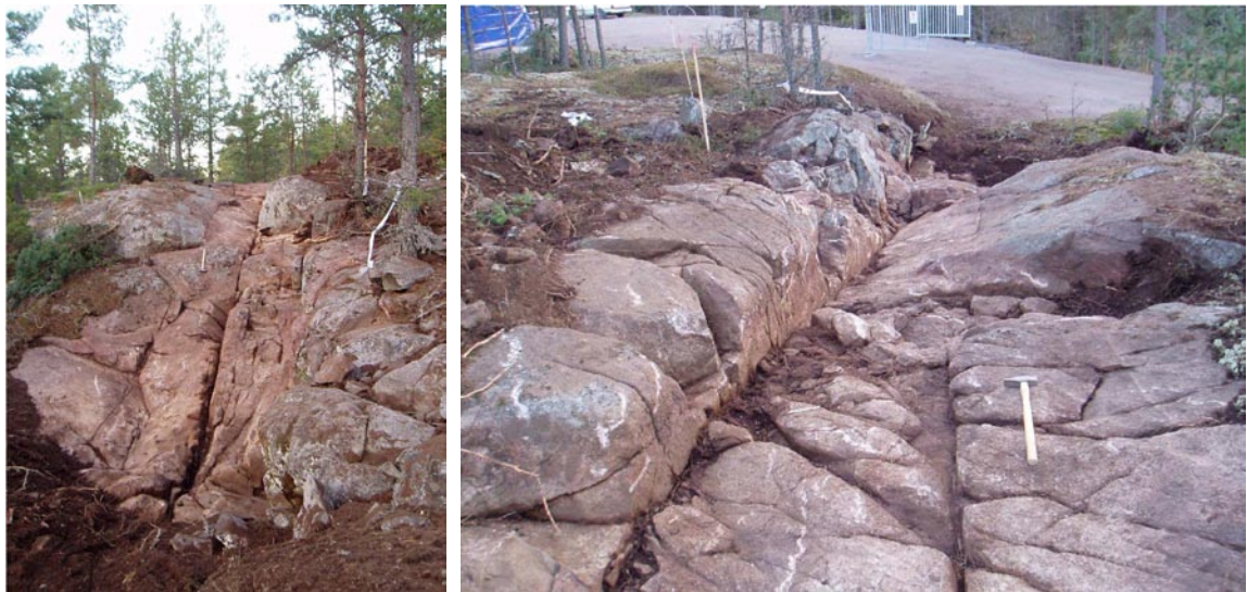
Figure 4-9. Photos of excavated rock around fracture zone MDZNS019A taken from north (left) and south (right), respectively.
