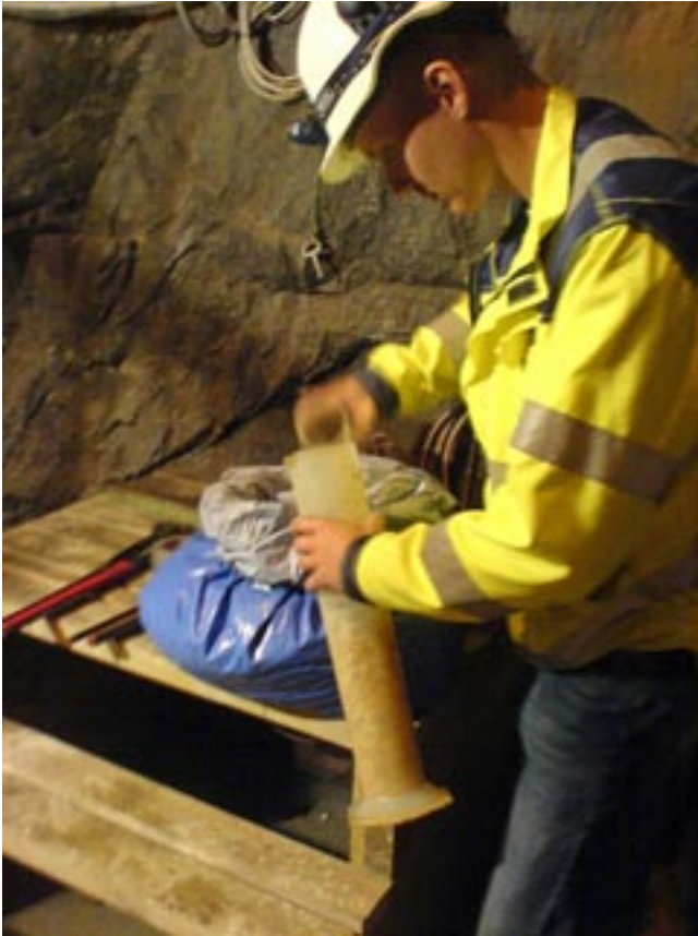
Figure 3-16. Pouring of pellets in cylinder with known volume for subsequent filling in borehole.
