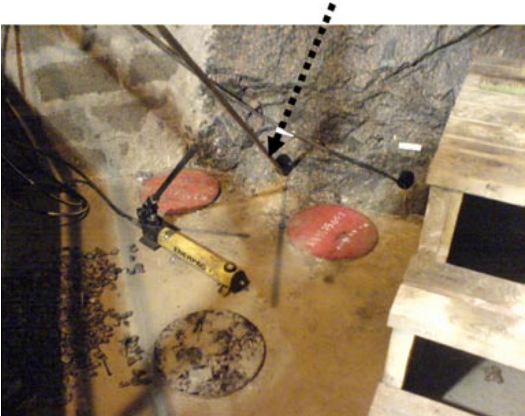
Figure 3-17. Rod with plate (dotted arrow pointing at it) for slight compaction of the pellet fill.
