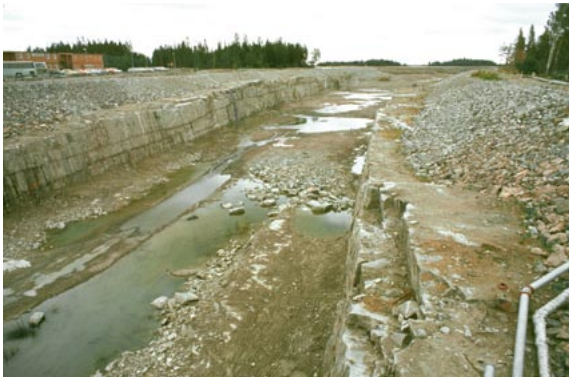
Figure 4-27. Picture from the construction of the 13 m deep and more than one kilometre long canal between the Baltic Sea and the nuclear power reactors. The horizontal fractures/ sheet joints are encountered along the entire excavation. There are several “beds” of extensive sheet joints on top of each other. The picture is taken from the southern side of the canal where the bridge crosses the canal between HFM20 and HFM22, see Figure 4-2. Reproduced from /Carlsson and Christiansson 2007/.
