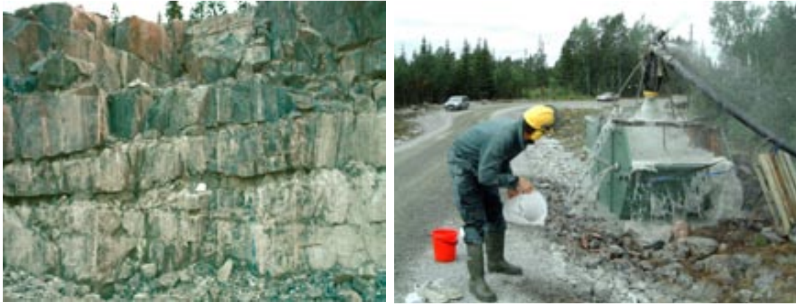
Figure 4-29. Two pictures of the near-surface bedrock in the north-western part of the tectonic lens (target area). The leftmost picture shows structurally dominant, but highly heterogeneous, horizontal sheet joints where the apertures are clogged by glaciofluvial sediments. This phenomenon is known to occur down to at least c. 50 m depth (KFM03A and HFM07) rightmost picture shows the flushing of a high yielding gently dipping deformation zone or sheet joint encountered at c. 40 m depth in HFM02.
