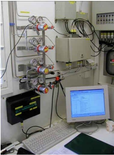
Photo 3. Computer room, displays and gas regulators.
