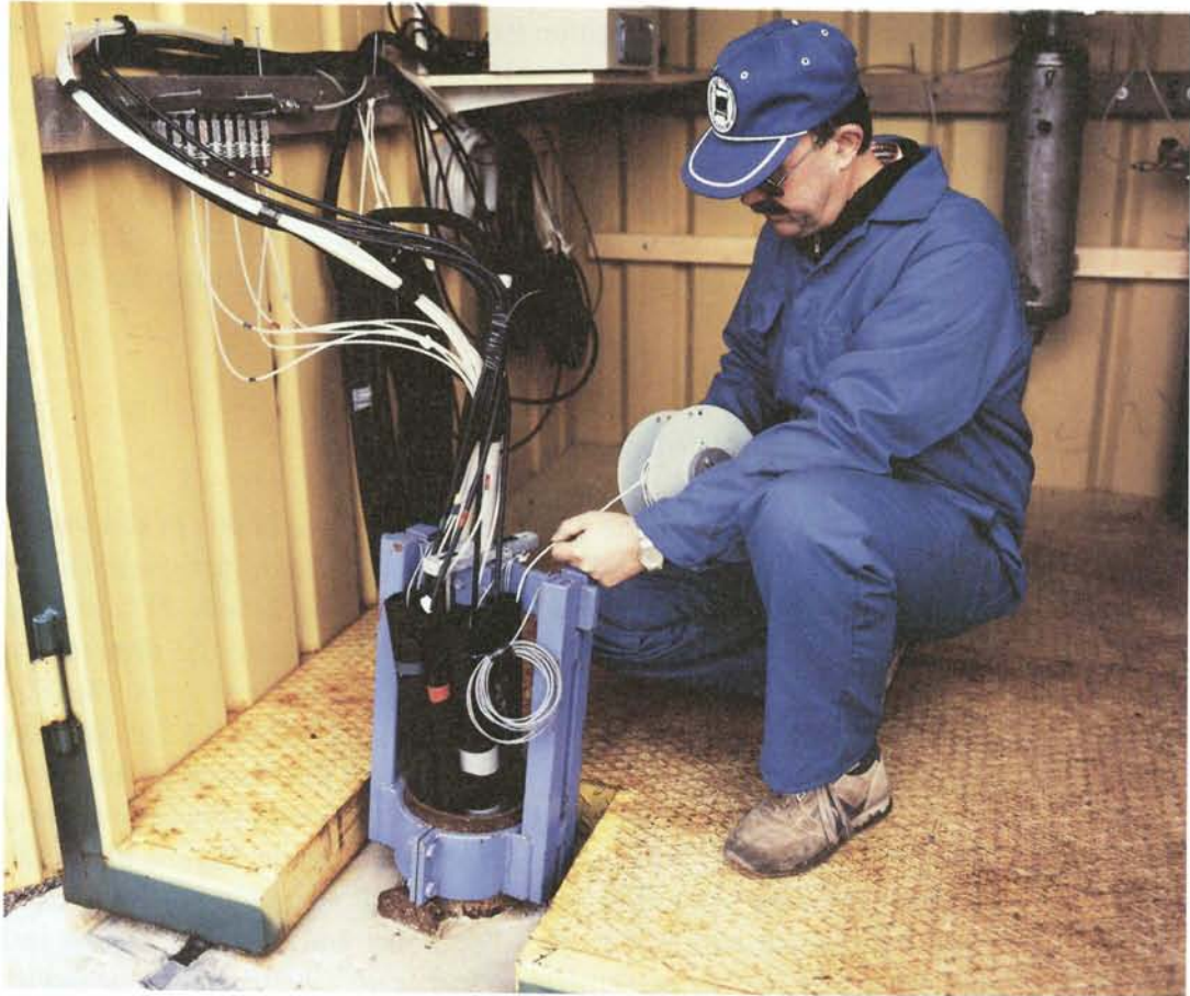
Figure 4-3. Top of monitoring borehole, showing bundles of pressure tubing, signal cables etc. Calibration of pressure recording is made by means of dipping a water level sensor in the stand-pipes.
