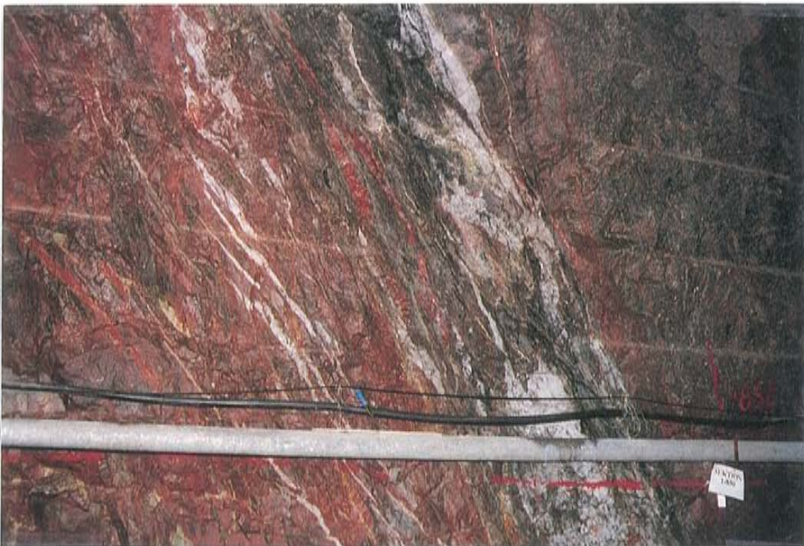
Figure 4-24. Fracture zone NE-2 at section 1844 m in the tunnel.
